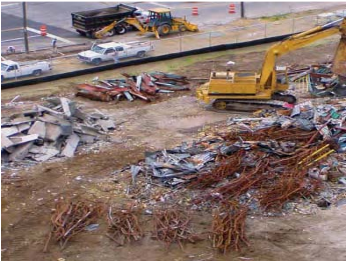
Figure 2.9: Different Types of Metals are Separated and Arranged at Demolition Sites for Recycling.
