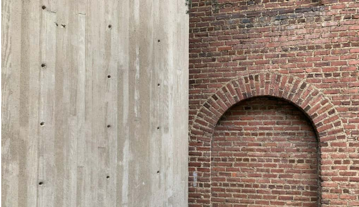
Figure 14: Detail showing the junction of M/G's addition to the original Penn Museum's bricks.
