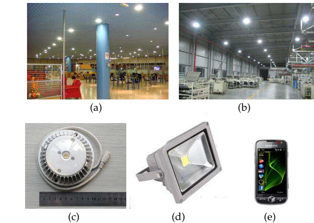
Fig. 1: LED lamps and light sensors. (a) LED lighting in an airport terminal. (b) LED lighting in a large warehouse. (c) An infrared LED lamp, 8 watts. (d) A high-power visible light LED lamp, 100 watts. (e) A smartphone with a light sensor (enclosed by red square).
